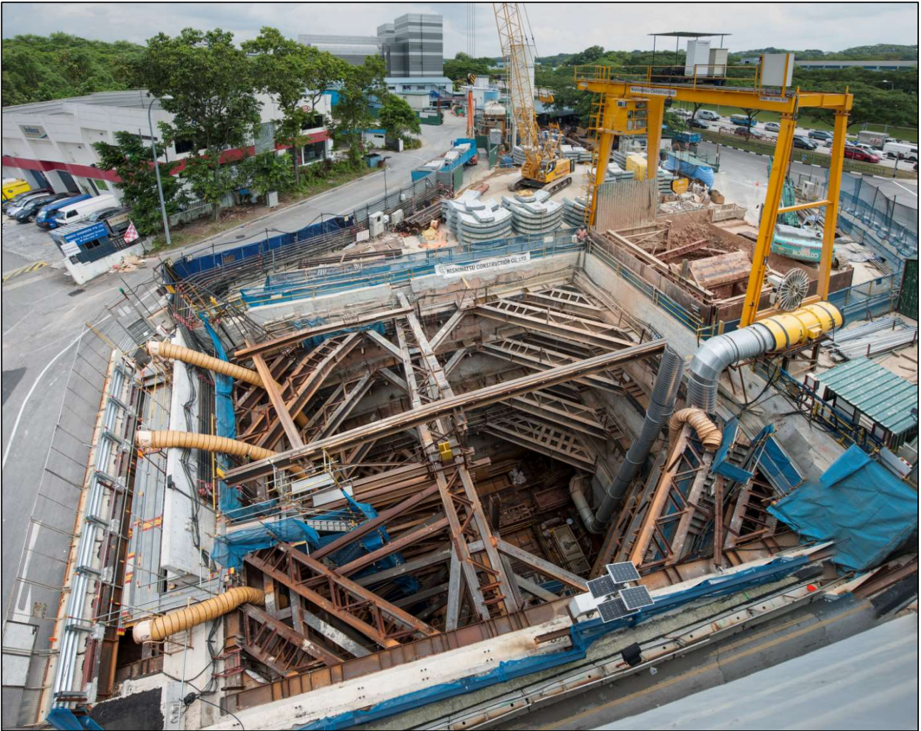
Figure 2-1: The gantry crane and the crawler crane can block each other's access to the shaft.
