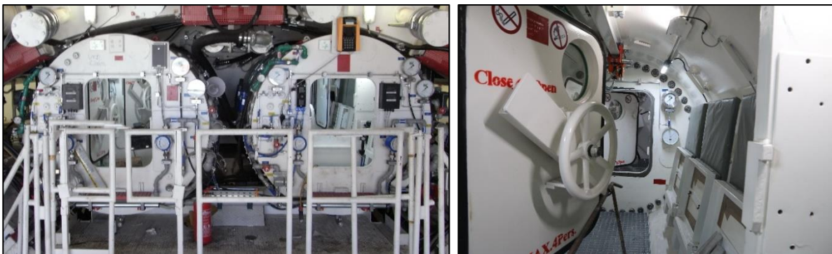
Figure 4-10: Air lock on the TBM for compressed air interventions.
