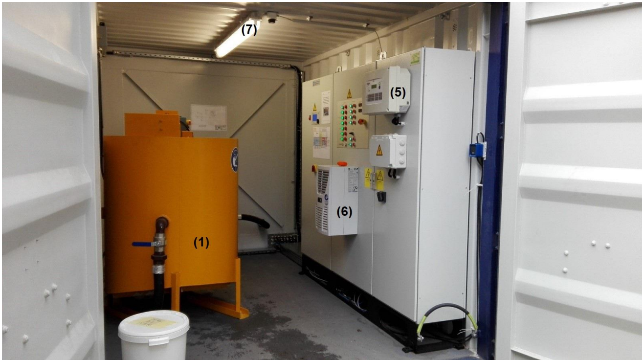
Figure 48: Control and mixing room: (1) stirrer, (5) control box for hydrogen sensors (6) air-conditioning device for cabinet, (7) illumination, (after Popovic et al., 2018)
