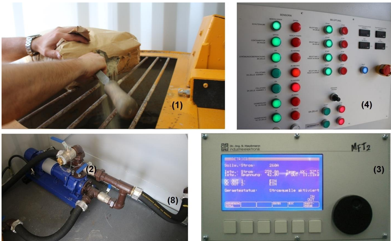
Figure 49: Content of the control and mixing room: (1) stirrer, (2) pump (3), DC source with control screen, (4) control panel, (8) pipes (after Popovic & Schößer, 2019)
